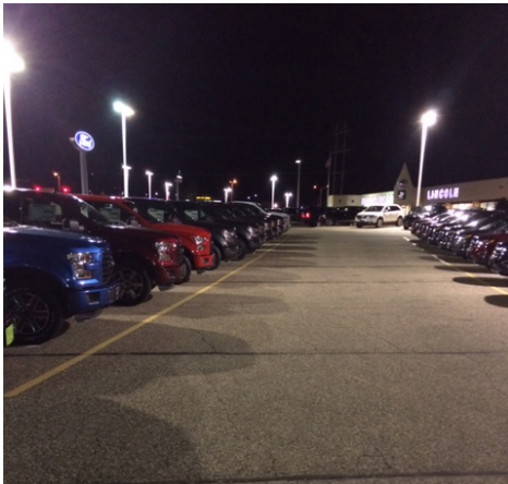
EXISTING Two - 1090W HID
