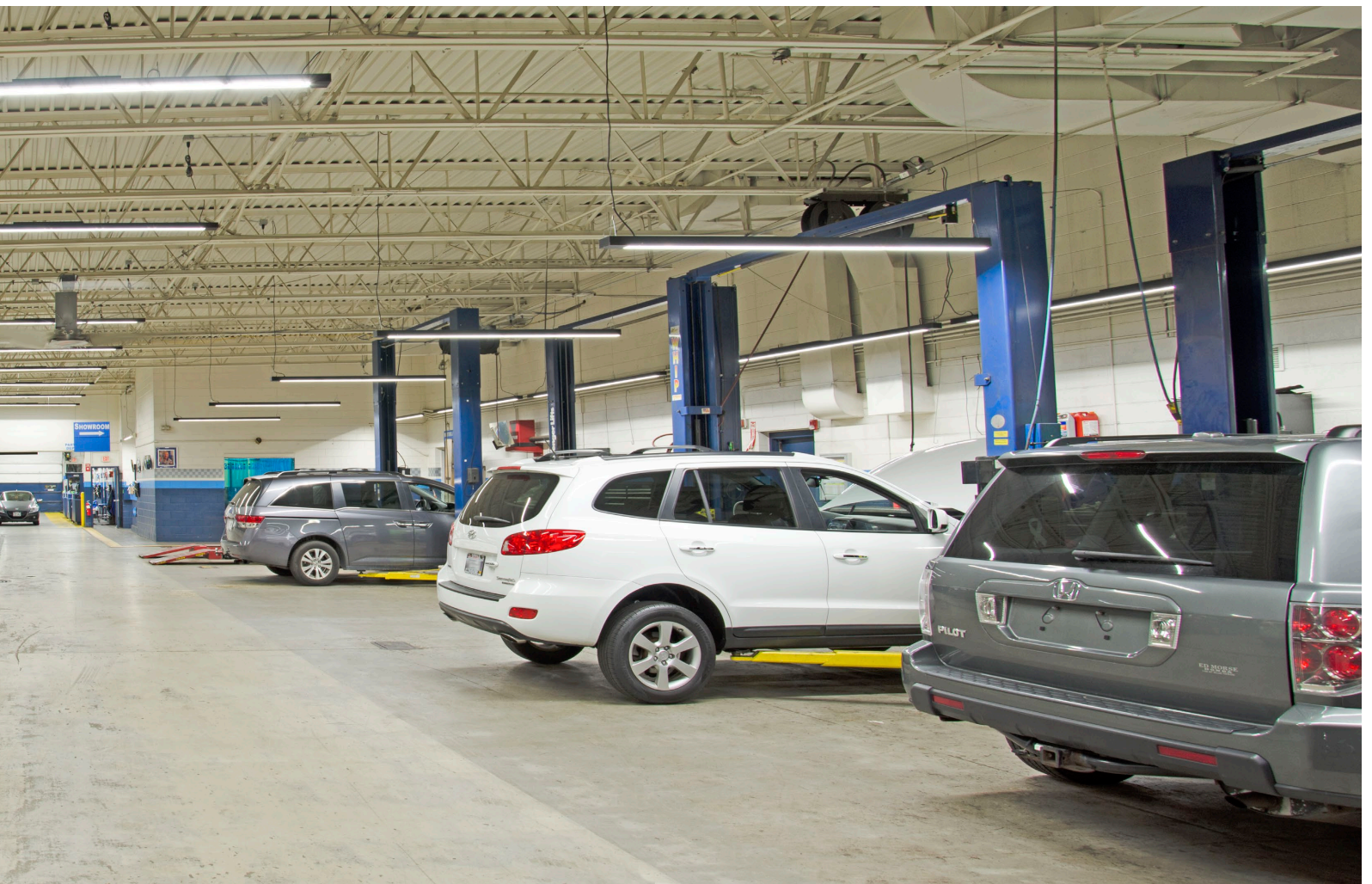
energybank Linear LED fixtures in the Service Bay area
